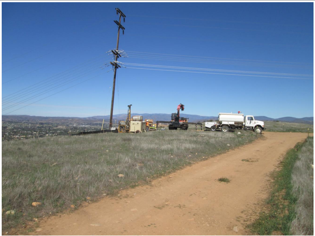
Photo 5: Crews were observed excavating at pole locations with fire watch/water tenders present within 50 feet of construction activity in accordance with the Project Fire Plan and APM HAZ-2.
