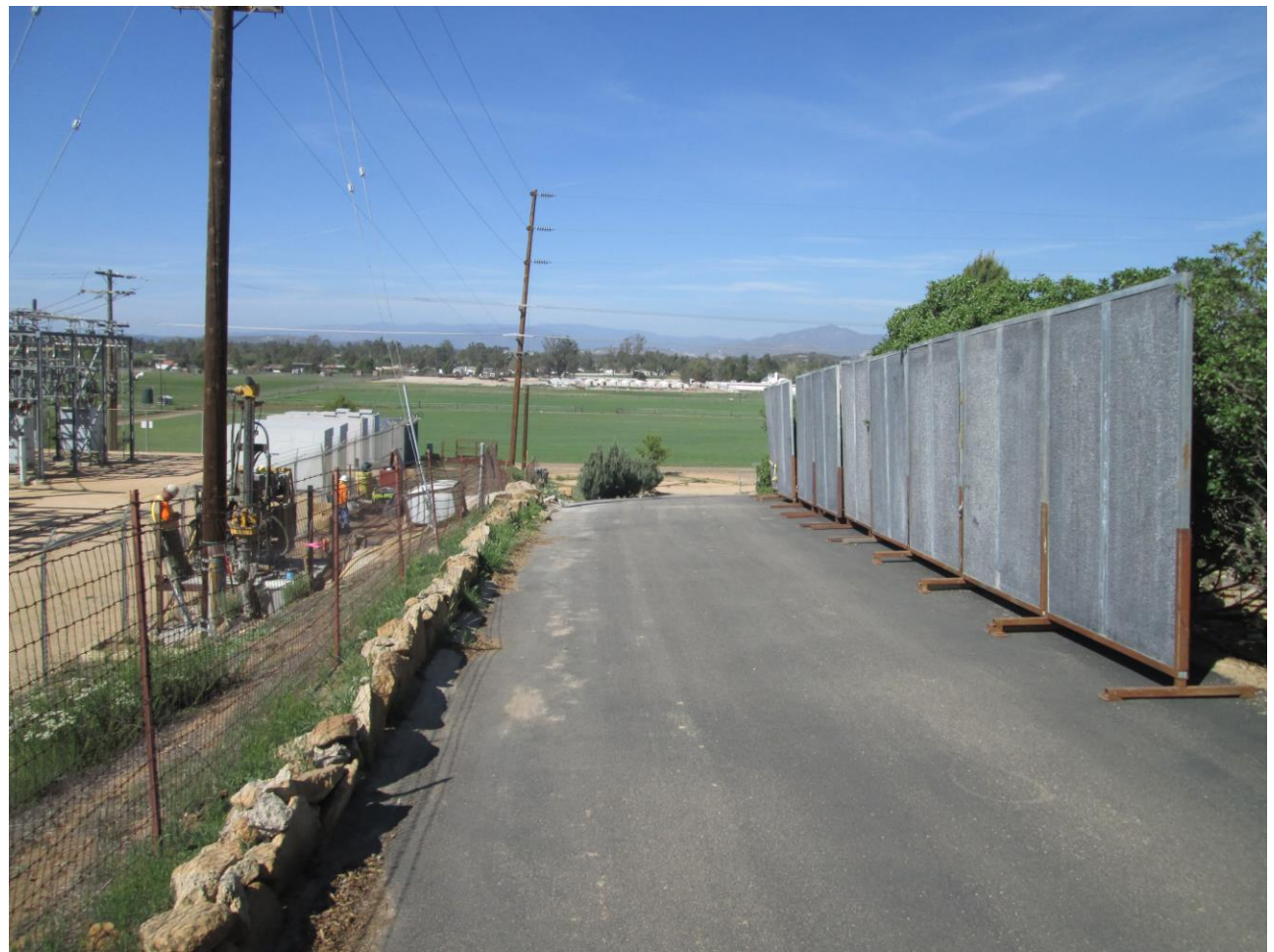
Photo 6: Noise Monitoring Equipment and sound walls were observed in place adjacent to micro pile drilling to ensure that noise levels during construction activities did not exceed thresholds at the nearest property line or adjacent to noise sensitive areas in accordance with MM NOI-1.
