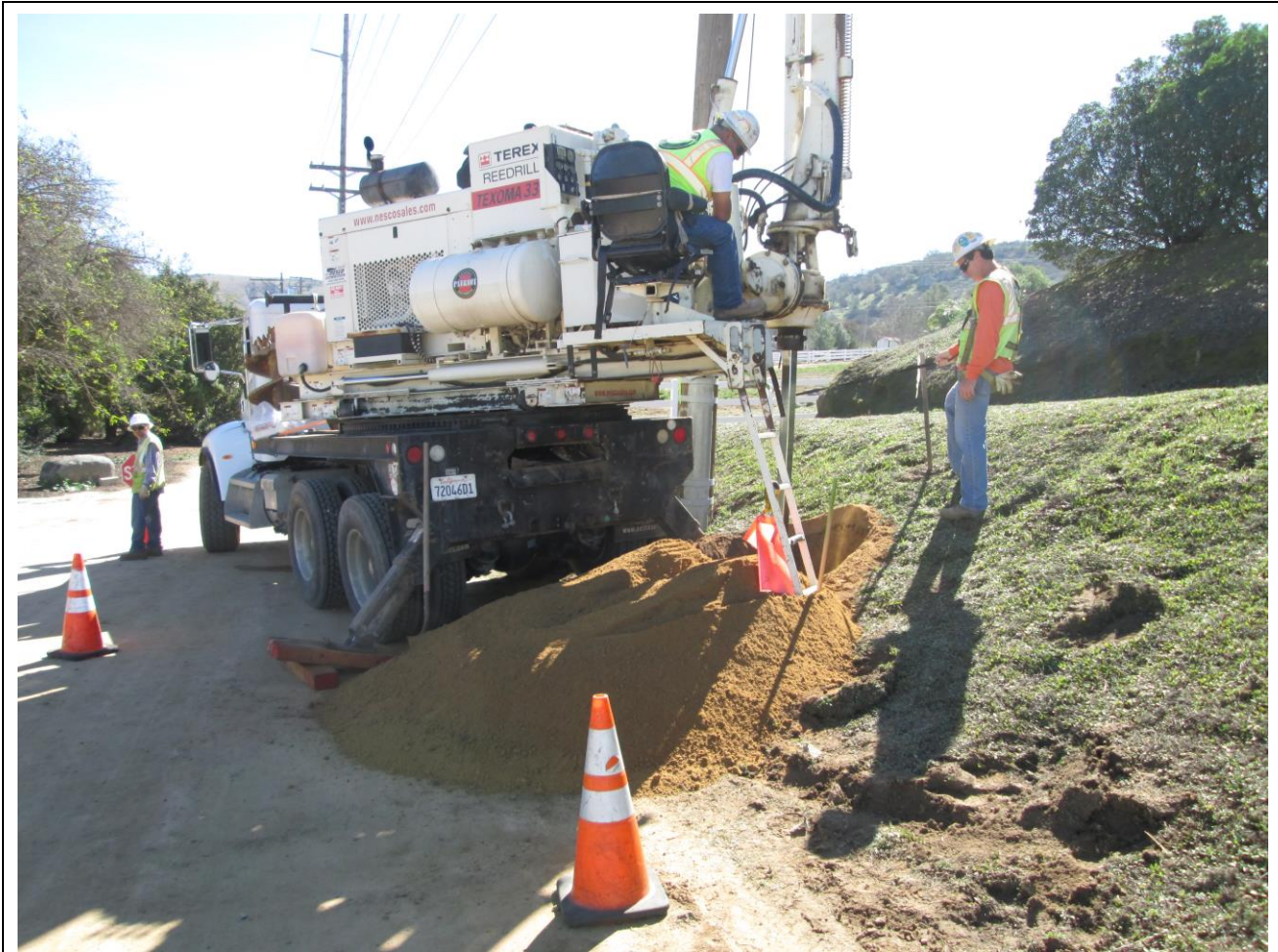
Photo 2: Crews were observed staging traffic control equipment (cones) and a flagger (left) during excavation work along Creelman Lane in accordance with APM TRA-1.
