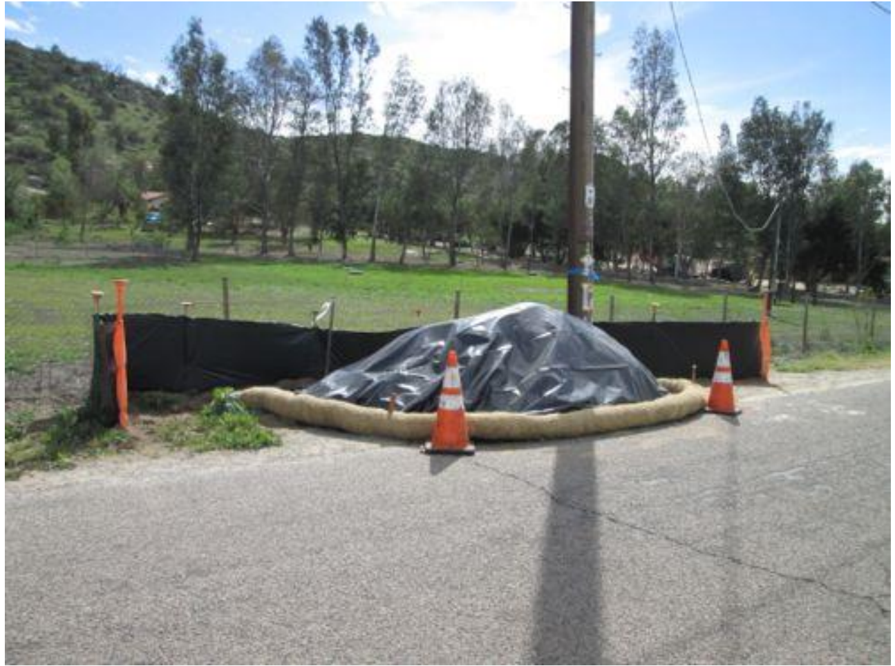
Photo7: Crews were observed placing visqueen in over spoil staged on site adjacent to a jurisdictional waterway in accordance with the project SWPPP and APM HYD-1. An aquatic resource monitor was on-site in accordance with the RWQCB Clean Water Act 401 Certification and MM HYD-4.
