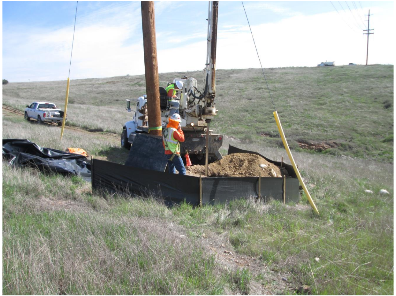
Photo 4: Paleontological monitors were observed inspecting excavated soils for the presence of fossils in accordance with APM CUL-6 during conventional pole hole digging. Excavated soil was contained by erosion- control silt fence in accordance with the Project SWPPP and APM HYD-1.
