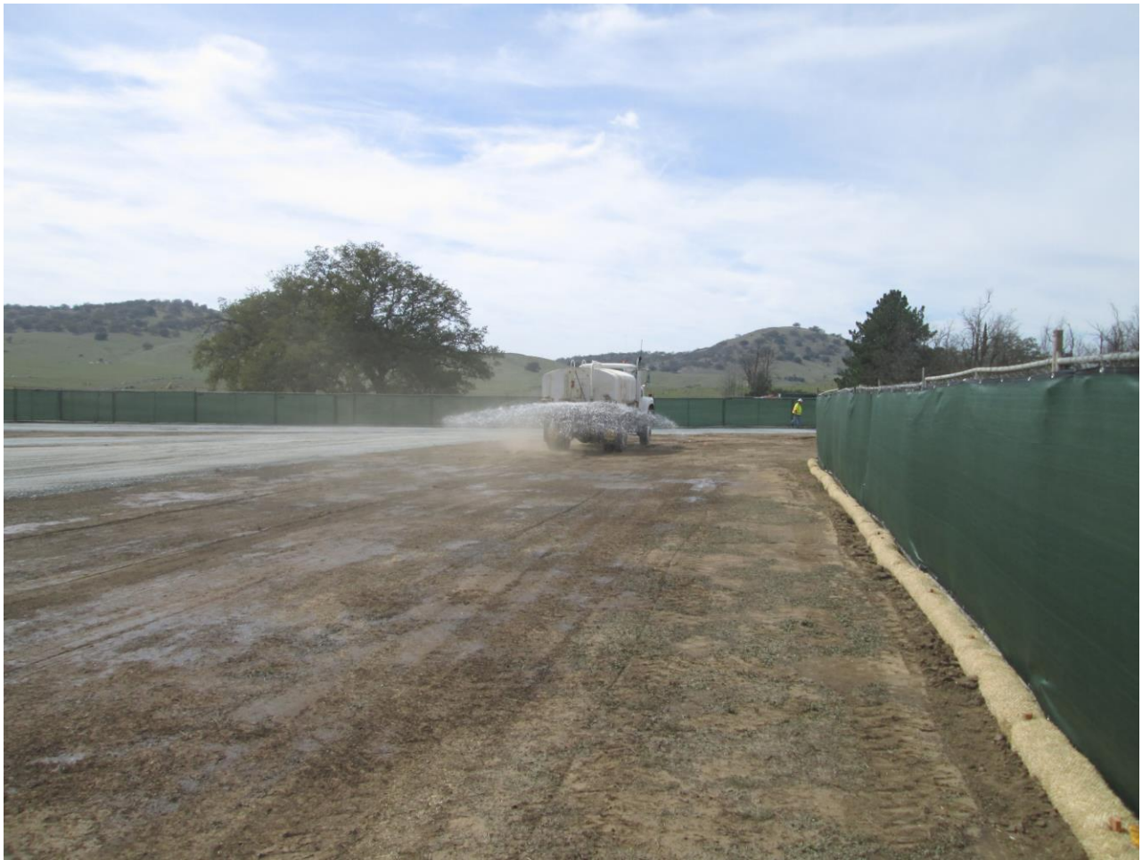
Photo 1: Opaque mesh screening material has been placed along the perimeter chain-link fence at the Santa Ysabel Staging Yard in accordance with APM AES-1. Straw Wattles have also been installed along the perimeter of the staging yard in accordance with the SWPPP and MM HYD-1. A water truck was observed applying water and preventing fugitive dust in accordance with APM BIO-1 during application of Class II road base.
